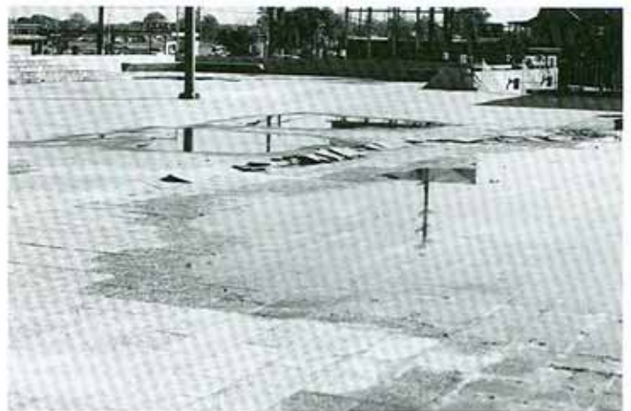
Improperly designed or constructed decks produce conditions leading to stain, efflorescence and exfoliation in any fascia material at their perimeters. In such extreme situations, damp-proofing as discussed in the text may fail, and physical isolation of the lower fascia from resultant leaks will be the only way to avoid problems.
